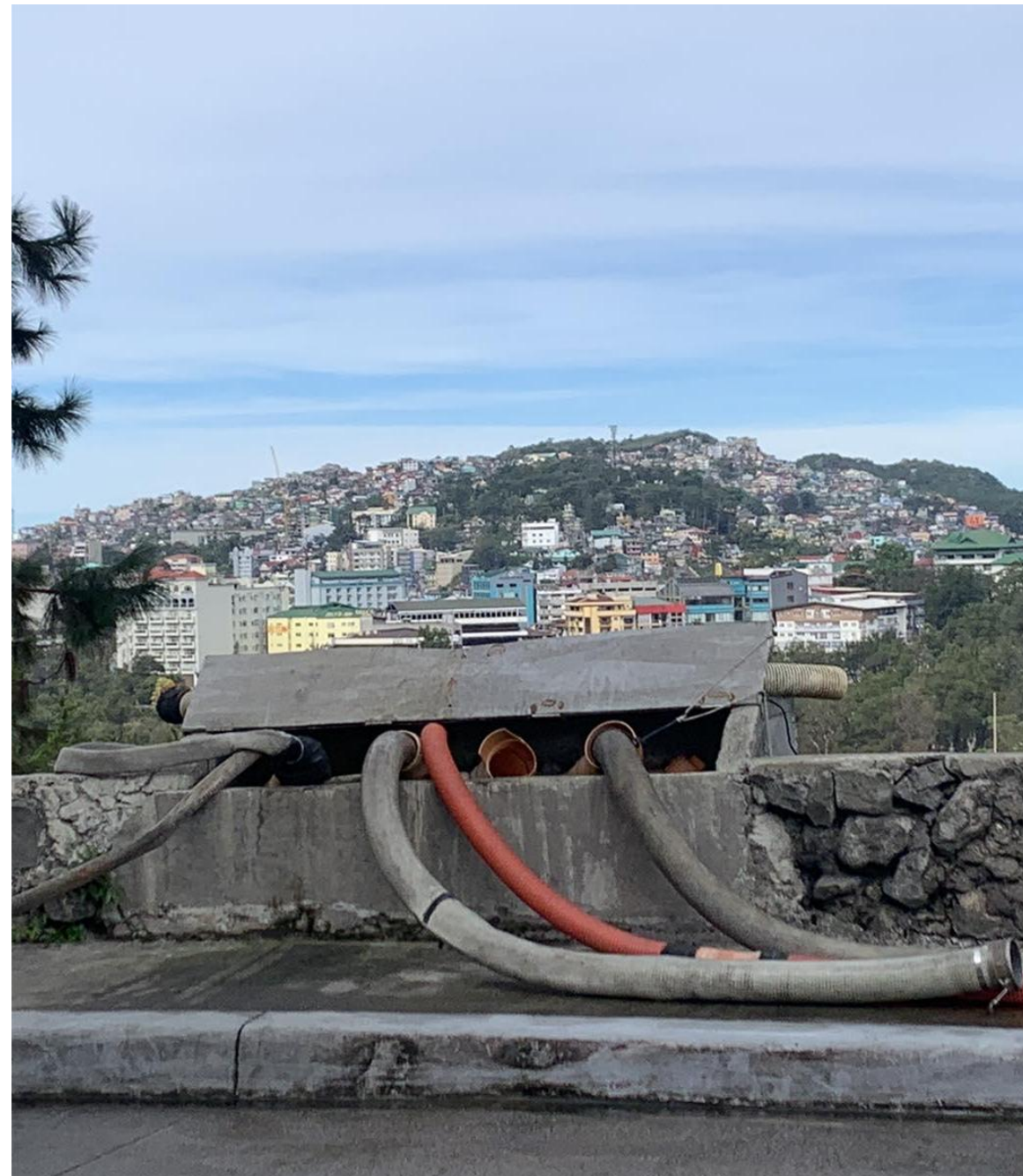
Uncovered water hoses going to cisterns
